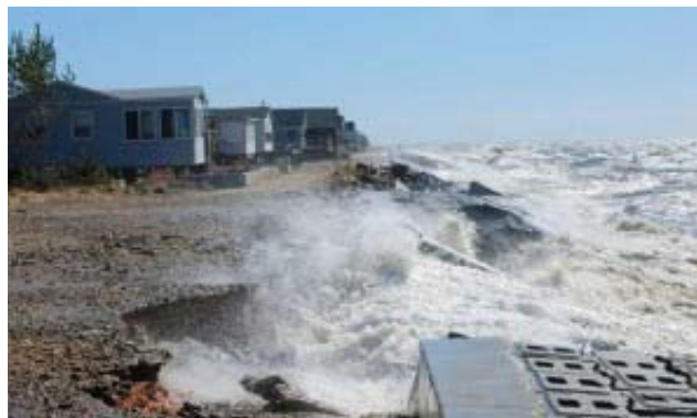
Undermined Seawall along Delaware Bay In Fairfield Township, NJ (Press of Atlantic City)
