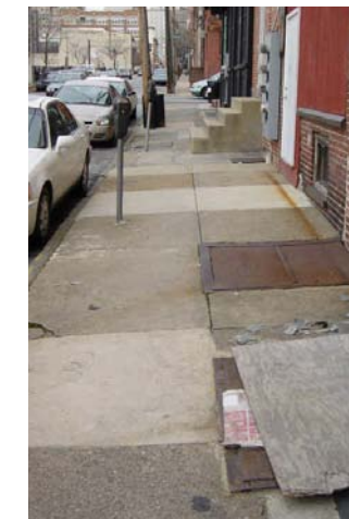
Undesirable Condition (existing) Uneven and peacemeal sidewalks throughout the corridor are unattractive. Underground vaults and their access doors will likely need to be replaced or painted to provide a consistent treatment.
