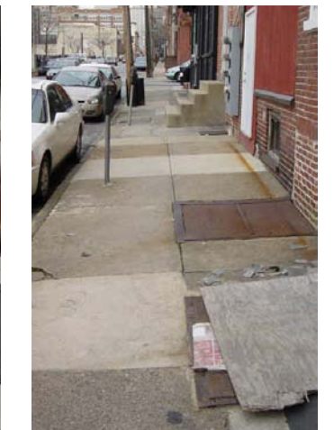
Undesirable Condition (existing) Uneven and peaceable sidewalks throughout the corridor are unattractive. Underground vaults and their access doors will likely need to be replaced or painted to provide a consistent treatment.
