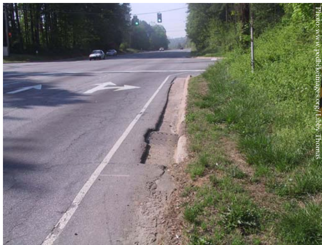
Broken pavement in the shoulder is unsafe and uninviting to bicyclists.
