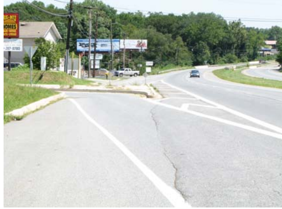
Pavement striping fronting the channelization island on US 40, near Sycamore Drive, interferes with bicycle traffic.
