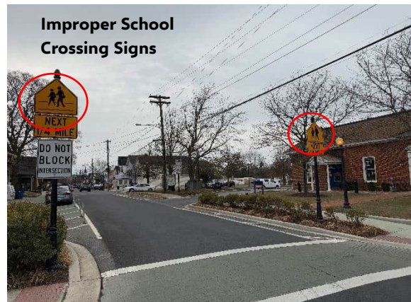
Figure 5.15: Improper School Crossing Signs SB MD 272
